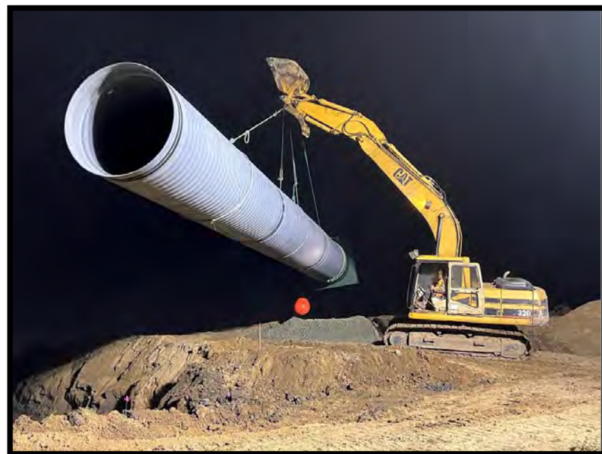
September 2023 – One of the double tide gates & culverts being moved to the installation location.
