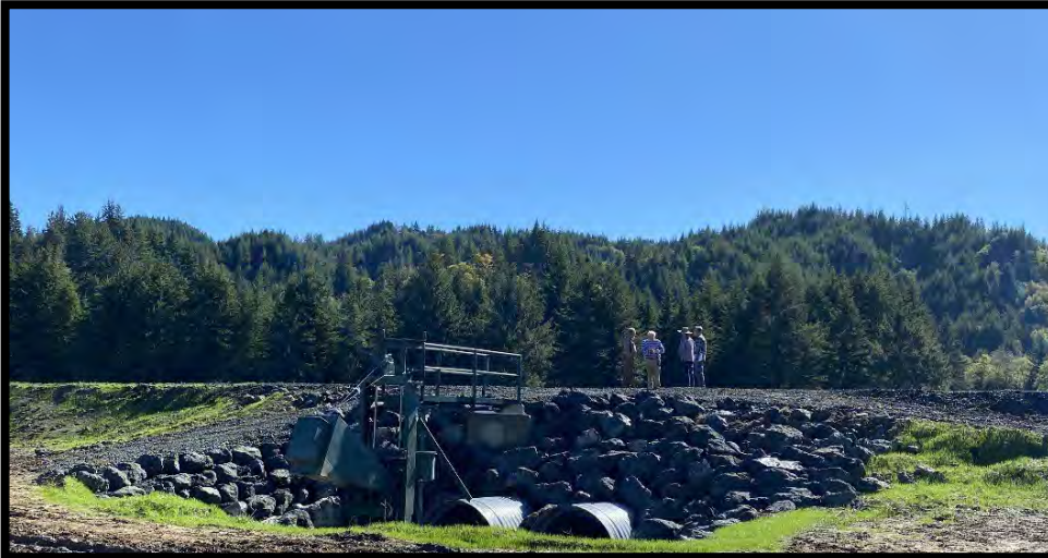
Interior view of MTR System with walkway installed on the left, and tide gate culverts installed on right.
